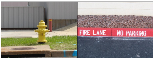
Unobstructed Fire Hydrant
